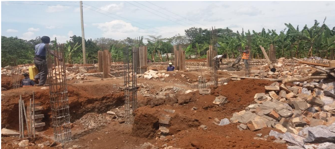
Photo 9: showing the Foundation after adjusting it to be fit for a stored building for offices near the new warehouse and office
